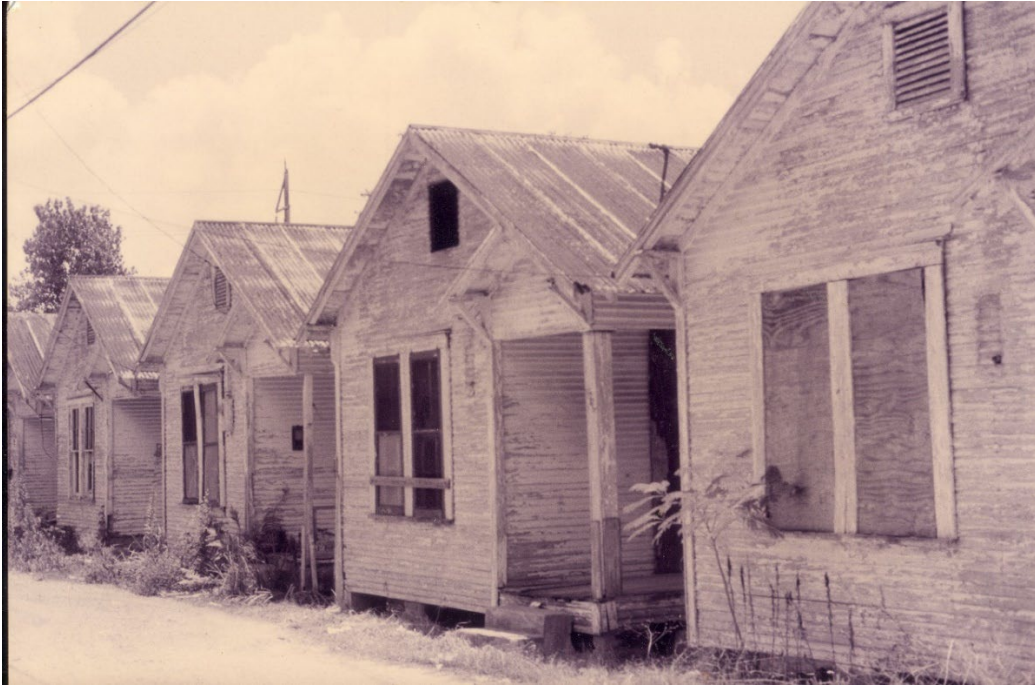
Figure 6 The original Row Houses prior to restoration. Photo by Sheryl Tucker Vasquez Courtesy of Project Row Houses
